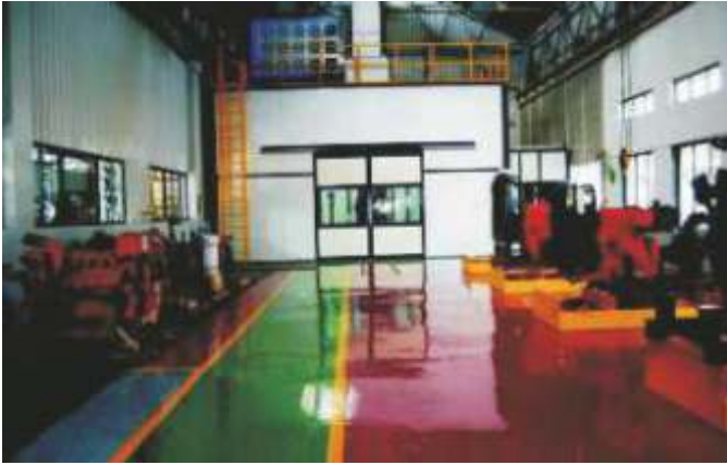
New state-of-the-art acoustic guard testing and packaging facility for FMUL fire fighting pumpsets at Kirloskarvadi
